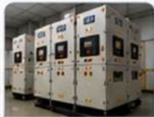
Capacitor Bank Installation
